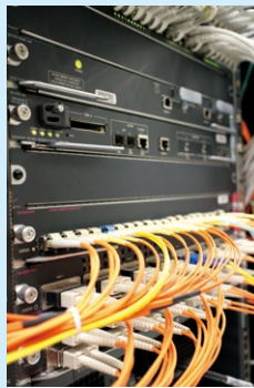
Cisco Catalyst 6509 core switch and 2960S switches in the Server Room
